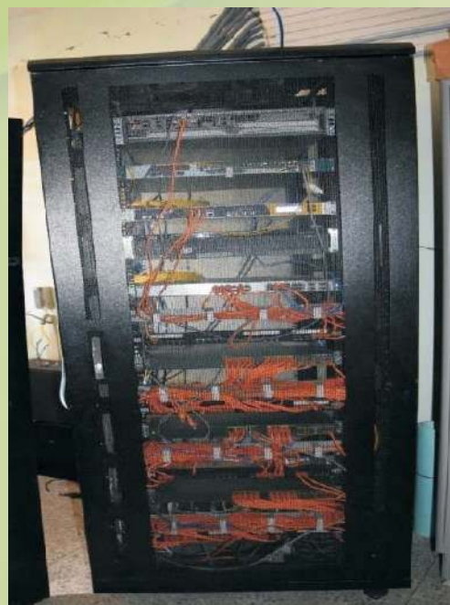
Firewall, Router Layered (L3&amp;L2) Switches
