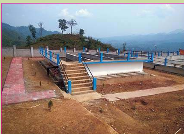
Water Supply System
