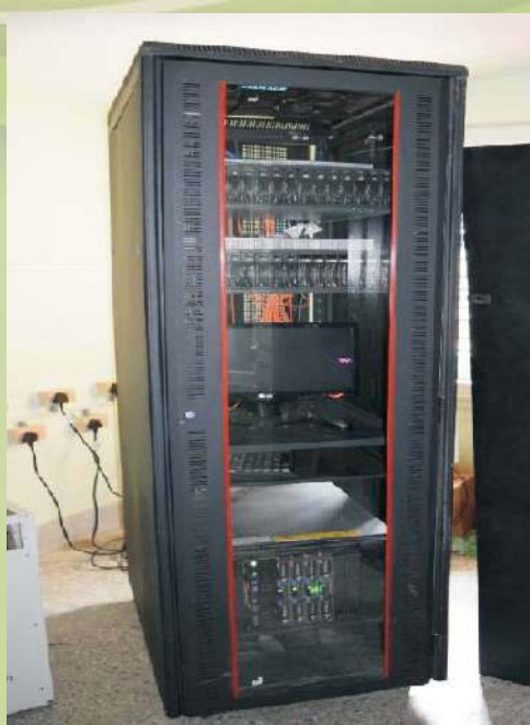
IBM Blade servers &amp; IBM Storage
