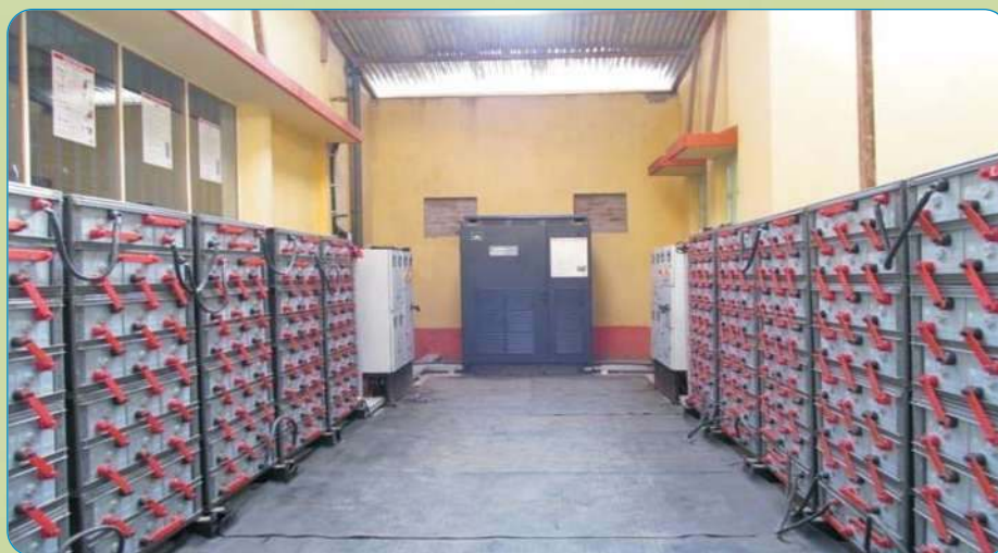
Solar Power Control Room
