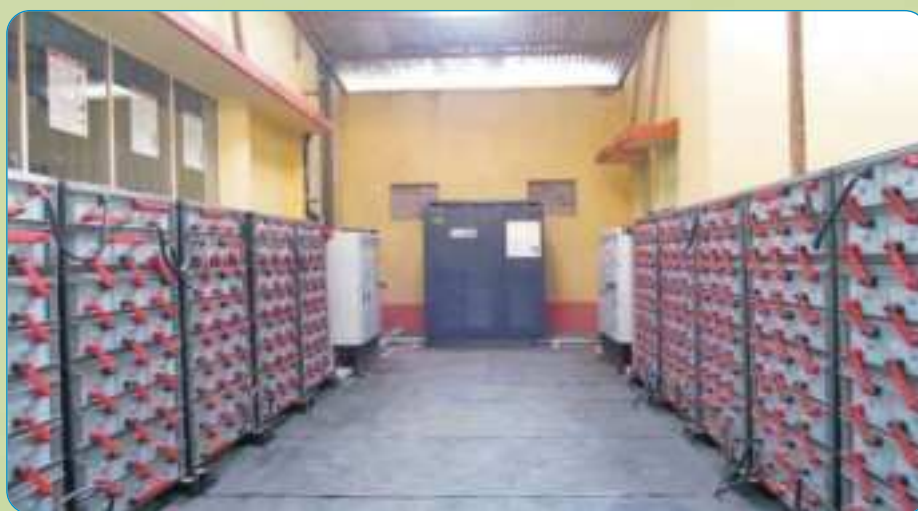
Solar Power Control Room
