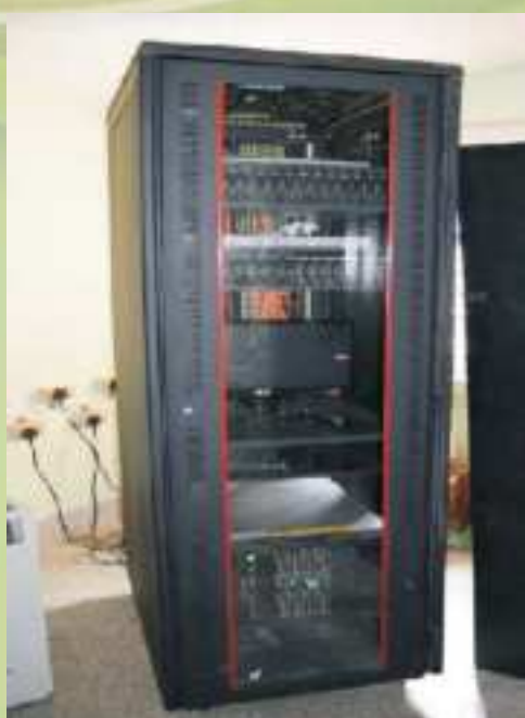
IBM Blade servers & IBM Storage
