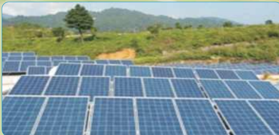
Solar panels of NIT- Arunachal Pradesh (This is reportedly the first of its kind among the thirty NITs)
