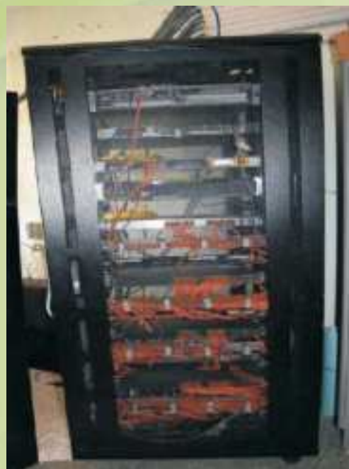
Firewall, Router Layered (L3&L2) Switches
