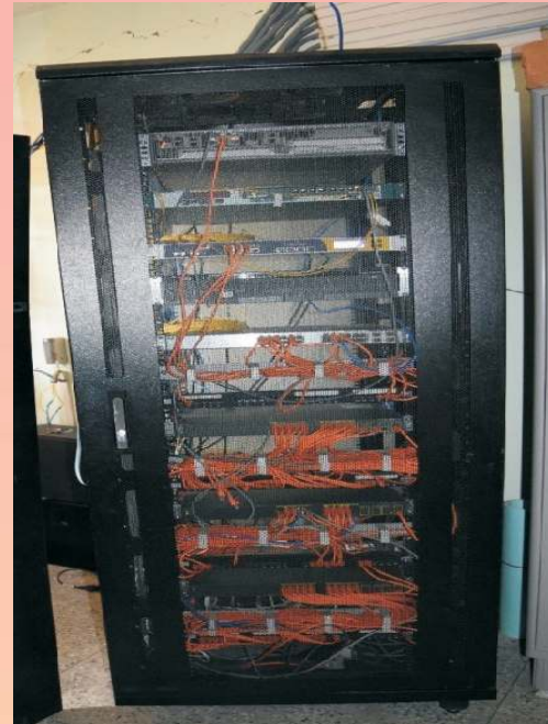
Firewall, Router Layered (L3&L2) Switches
