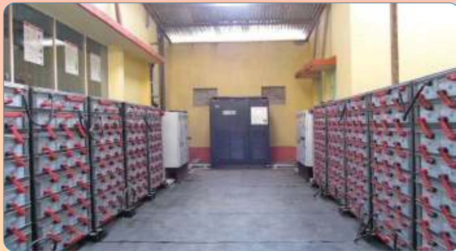
Solar Inverter and Battery back-up
