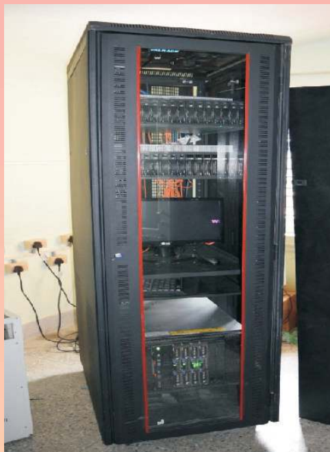
IBM Blade servers & IBM Storage
