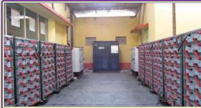
Solar Inverter and Battery back-up
