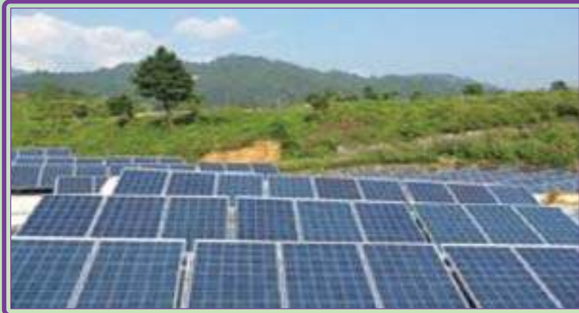
Solar panels of NIT- Arunachal Pradesh [This is reportedly the first of its kind among the thirty (30) NITs]
