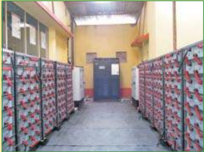
Solar Inverter and Battery Back-up
